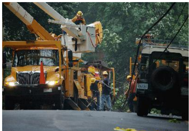
Contractors work to repair a power line that was taken down by a tree in Northern Virginia after a summer storm.
