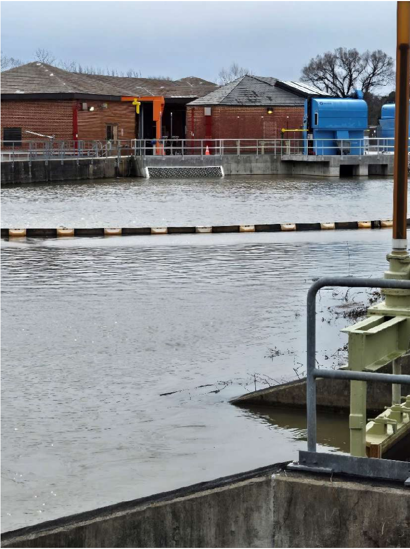
Figure 7. Raw water basins
