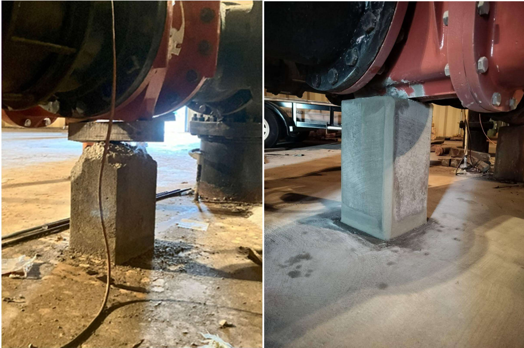
Figure 29. Wood supporting valve due to eroded concrete support (2025), Support repaired (2026)
