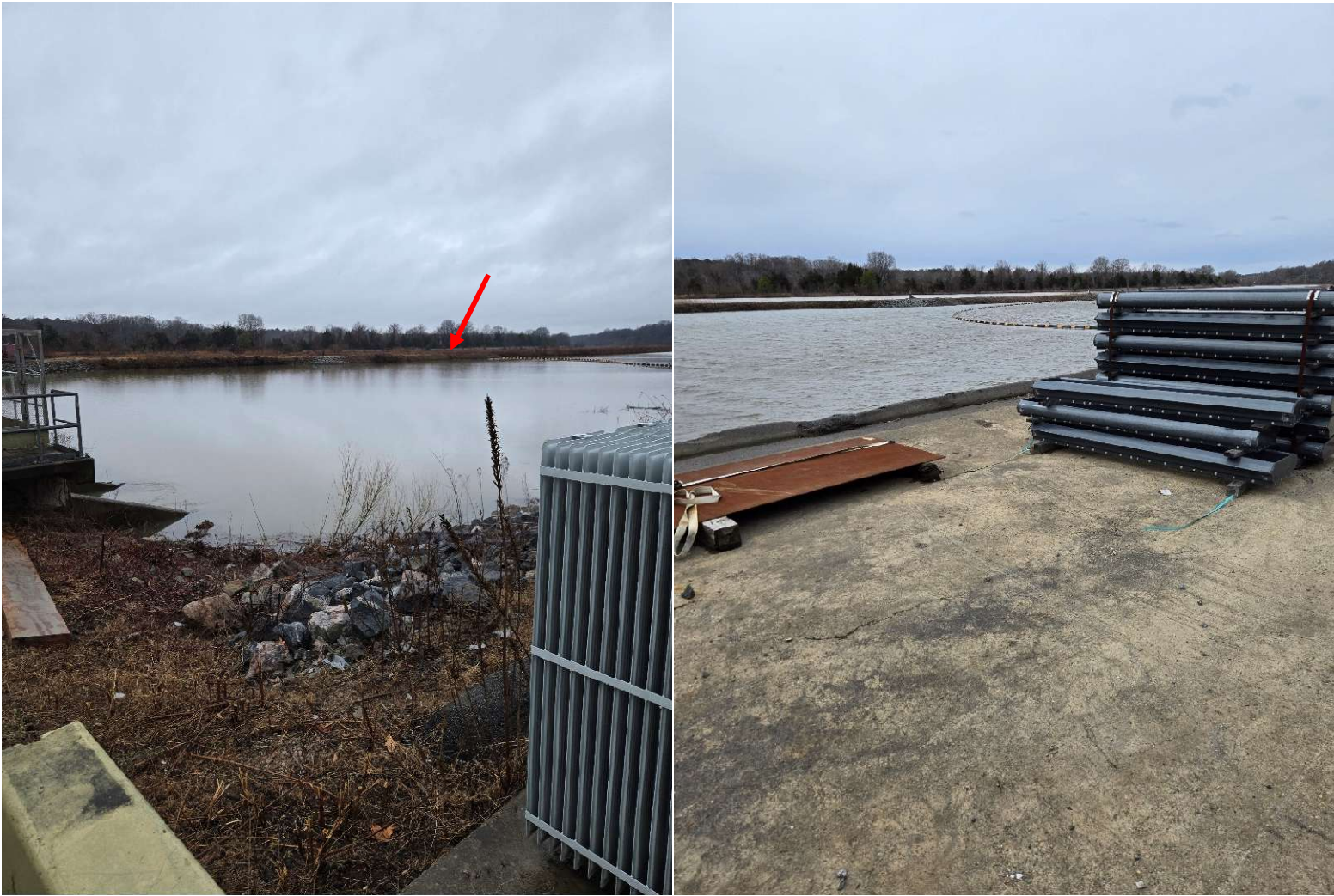
Figure 6. Earthen berm between lagoon and raw water intake channel (2025 left), Shrubs less growth observed (2026 right)
