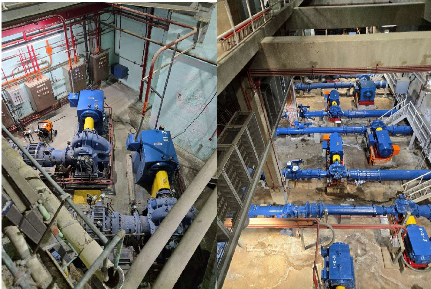
Figure 28. Korah Pump Stations
