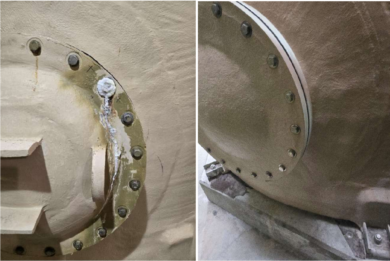
Figure 24. Chemical leaks (2025), Not observed (2026)
