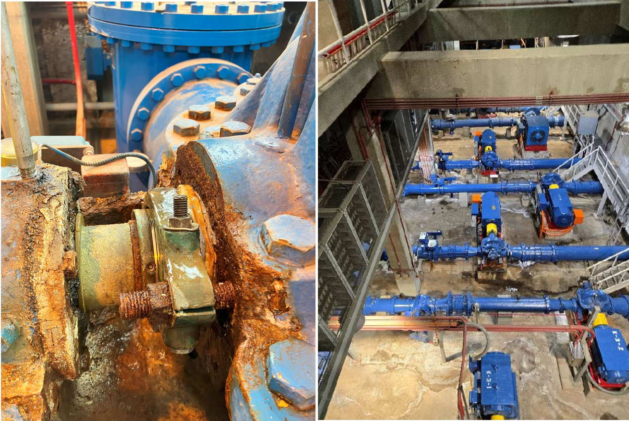
Figure 30. Corrosion at several pumps (2025), Pumps painted and no visible corrosion (2026)
