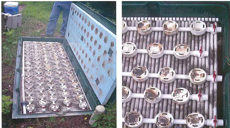
Photograph 6: AdvanTex ® System Receiving Residential Effluent with No Water Softener Backwash
