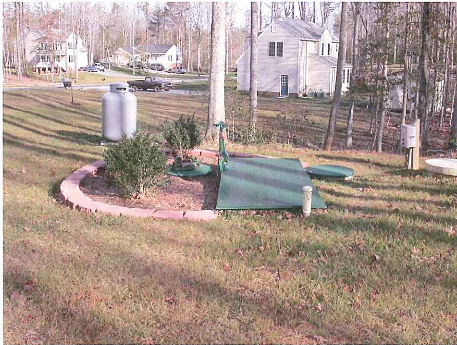
Photograph 1: Typical AdvanTex® Installation
