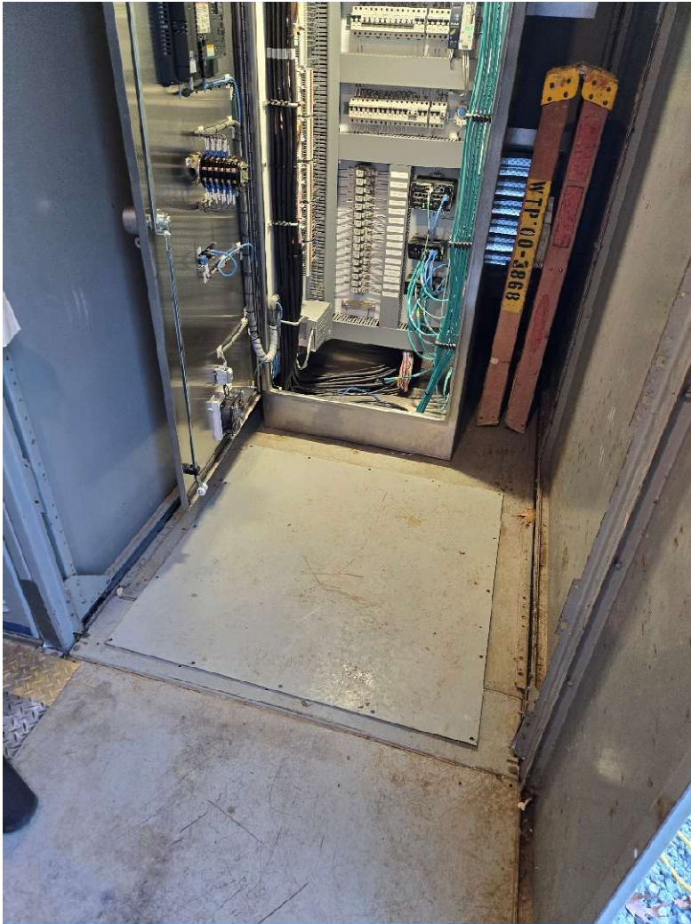
Figure 2. Automatic transfer switch installed
