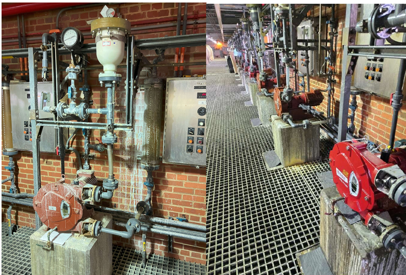
Figure 25. Chemical leaks (cont.) (2025), Not observed (2026)
