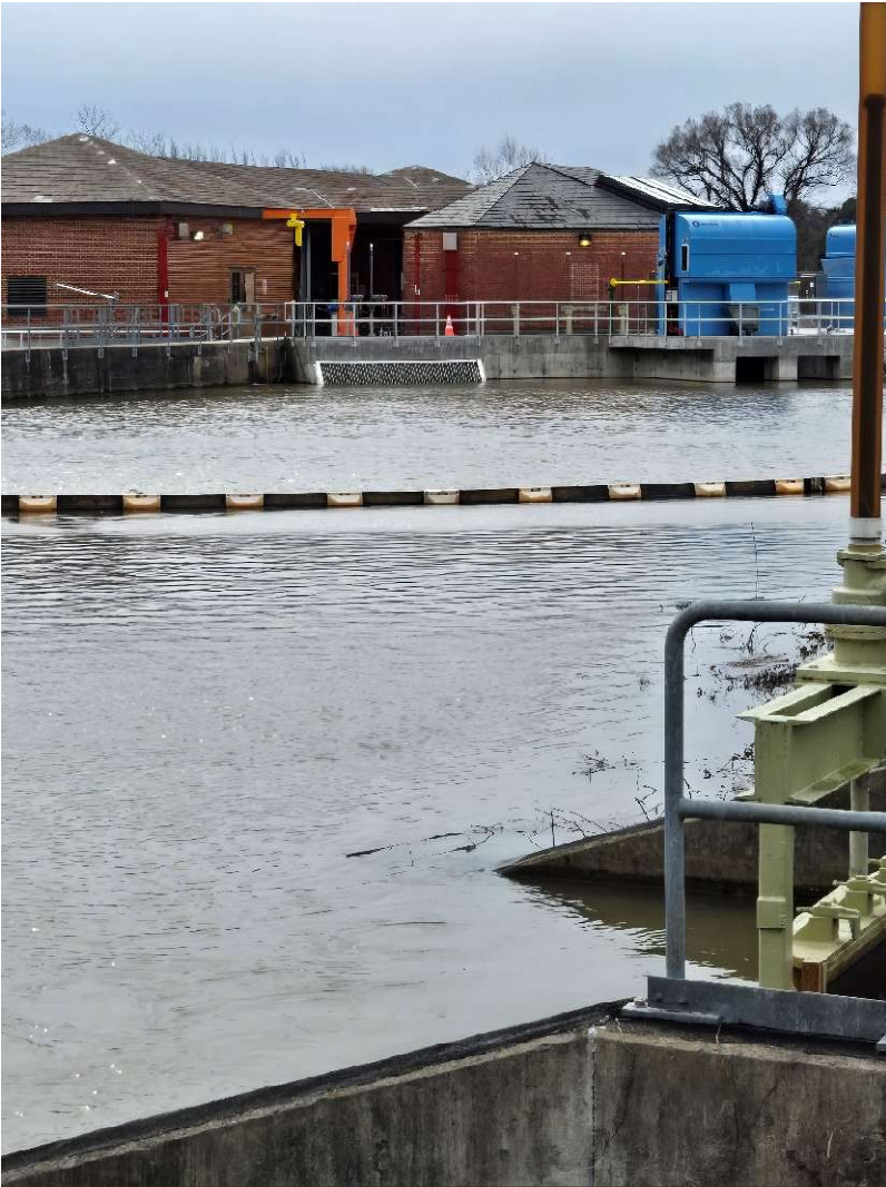
Figure 7. Raw water basins
