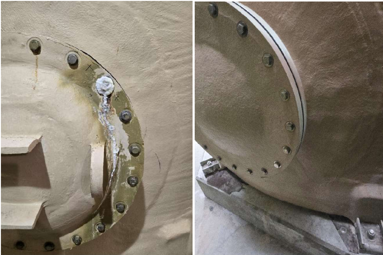
Figure 24. Chemical leaks (2025), Not observed (2026)
