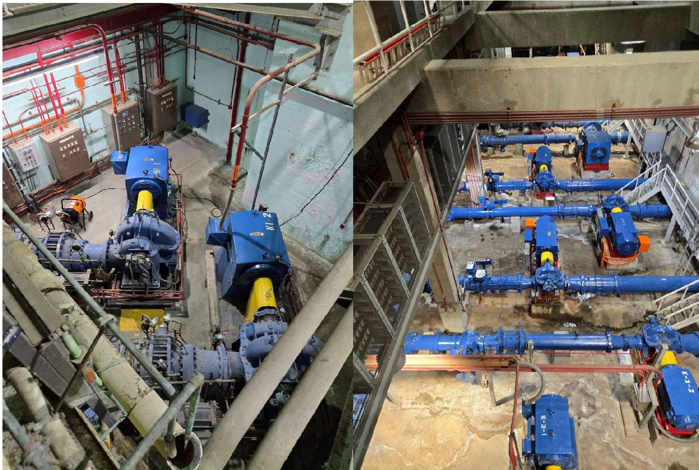
Figure 28. Korah Pump Stations
