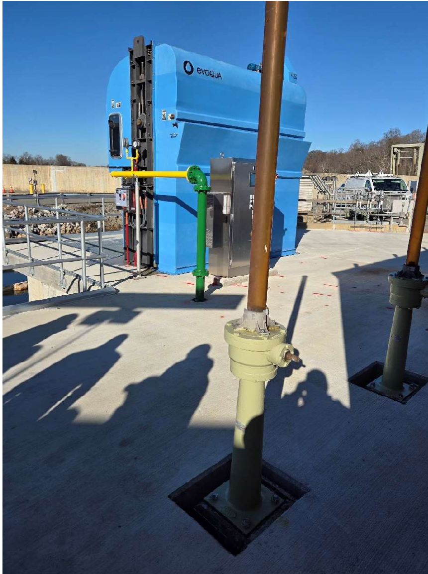
Figure 8. New raw water screens
