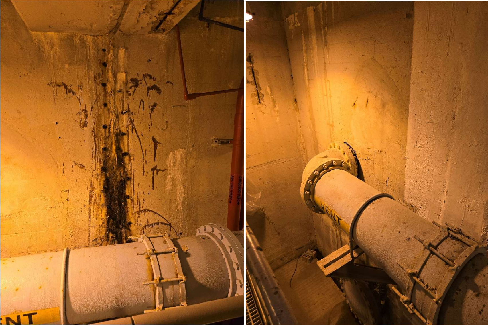
Figure 17. Leak and biological growth (2025); No leak observed (2026)
