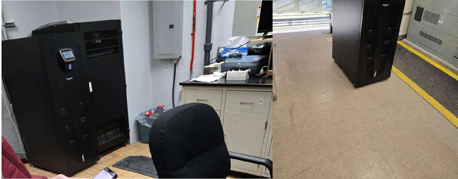
Figure 3. UPS systems upgraded. Plant 1 (left), Plant 2 (right)
