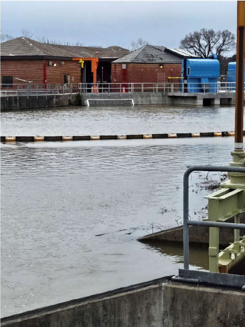
Figure 7. Raw water basins
