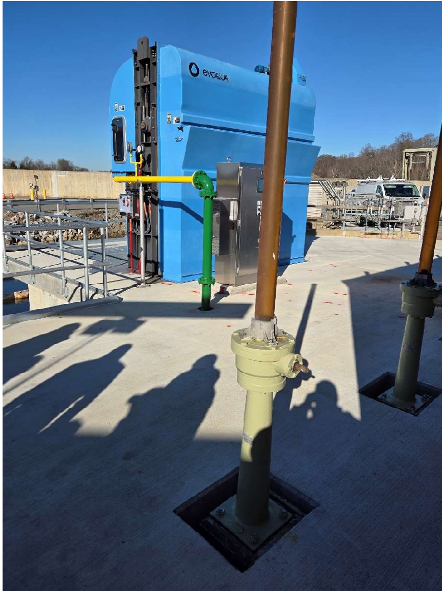
Figure 8. New raw water screens
